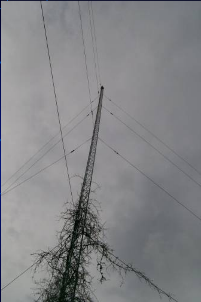
Damaged 160M vertical
